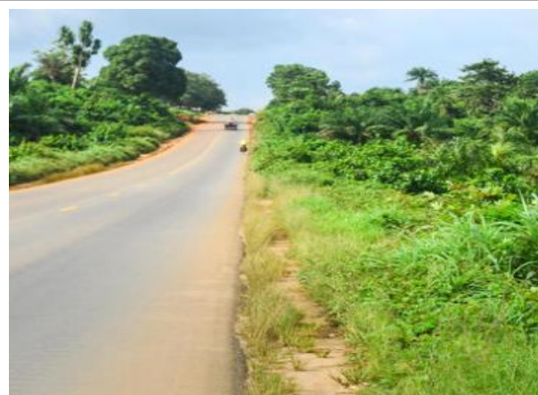
Figure 18: View of the condition of the Monrovia to Tubmanburg road
