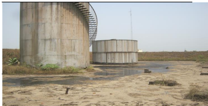
Figure 14 Visible hydrocarbon contamination at Port
